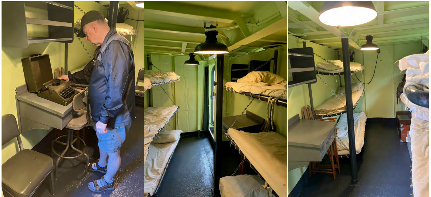
TOP ROW: Painters are John Ragno and Jay Hoag. A desk got a new coat of paint. Steve Adams and Jerry Gilmartin installed the bunks.
